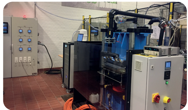
ITM power PEM electrolyser used for grid service tests at DTU
