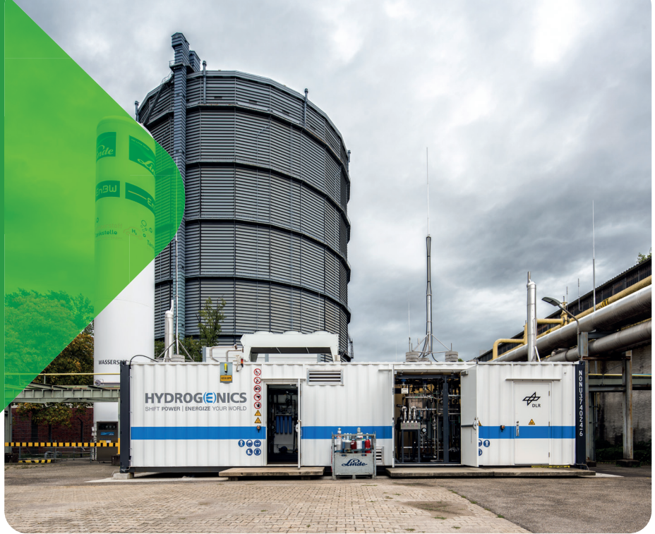
Container-integrated PEM electrolyzer linked to a H2 refuelling station used at DLR for grid service testing
